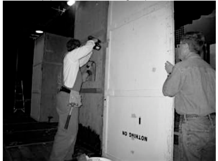
Ben Hohman and Harold Warren attaching more panels to build the wall.
