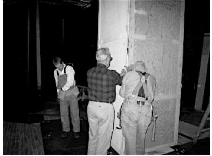
Ben Hohman, Ed Jahn, and Don Stubb putting up panels on the wagon platform.
